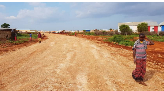
Completion of feeder road in Baidoa. Photo: Abdullahi Abdulle, Livelihoods Project Officer, Danwadaag Durable Solutions.
