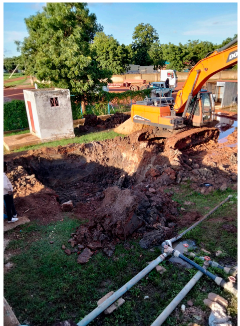
Excavation for foundation of pressed steel tank in Bentiu Water treatment plant, Rubkona County, July 2022. Photo: Stephen Waswa Otieno / Concern Worldwide.
