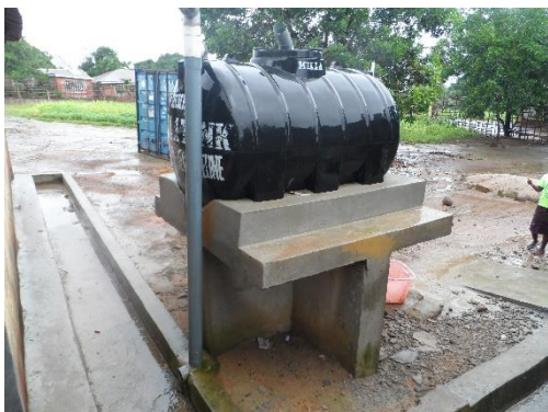
Figure 2: Example of a rainwater collection tank from a health care facility roof in Sierra Leone (John Heelham)
