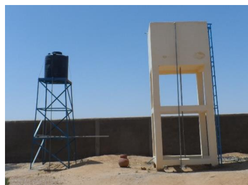
Figure 1: Example of a raised water tank at a health care facility in Chad (John Heelham)
