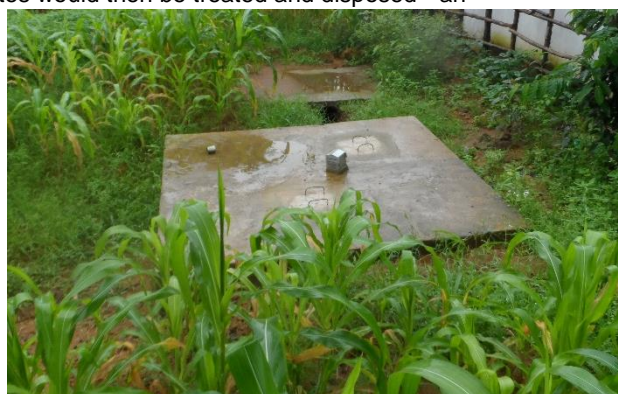
Figure 3: Example of a lined, protected pit for infectious waste in Sierra Leone (John Heelham)
