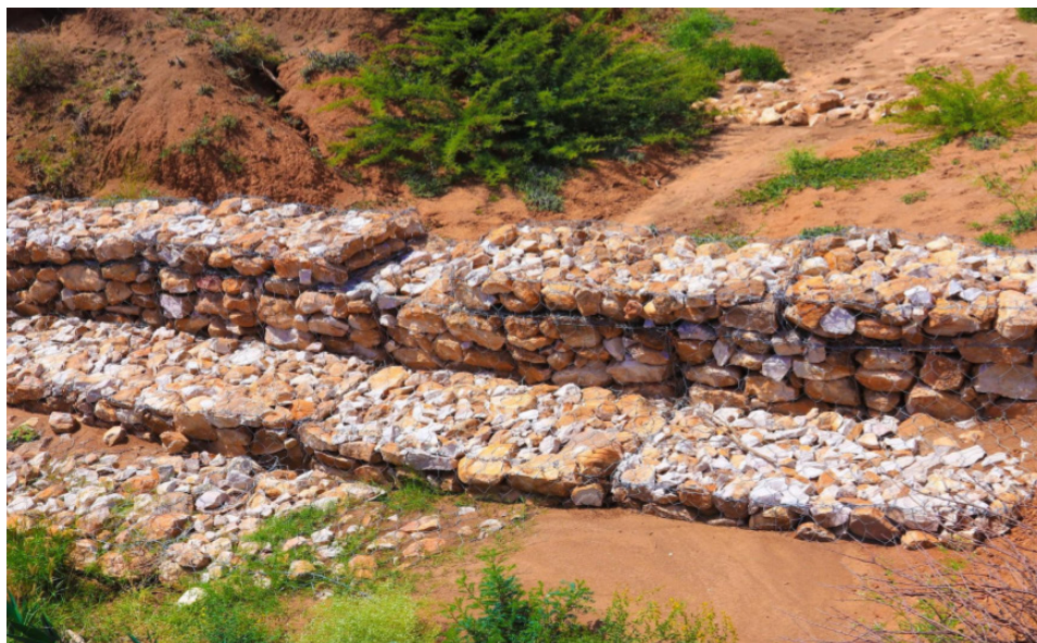
Figure 2: Gabion check dam near Korji village, Gabiley, Somaliland. The dam ledges shown above assist the accumulation of soil behind the gabions. Photo: Mohamed Ahmed Ibrahim/Concern Worldwide.
