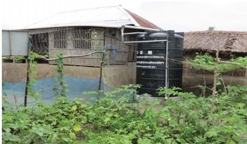
Integrated model of Household level Rainwater Harvesting System with vegetable gardening in coastal area
