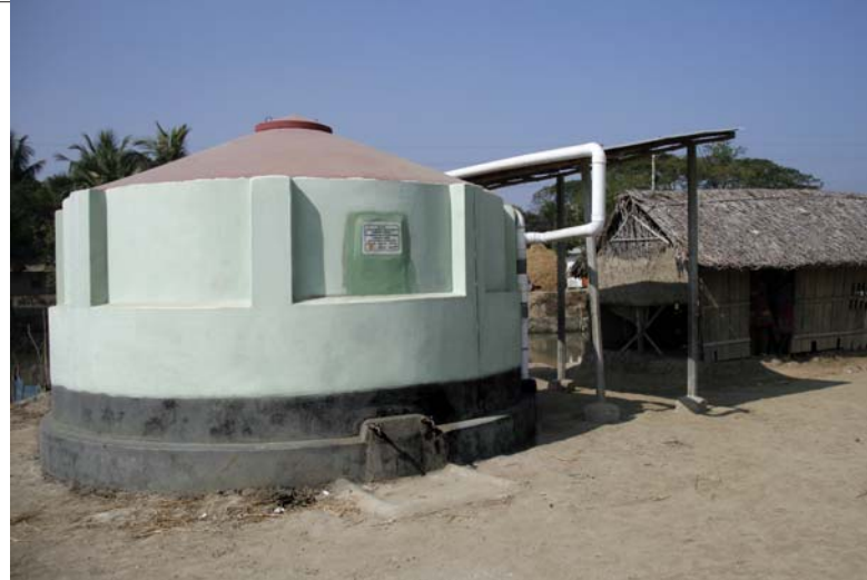
A school based Rainwater Harvesting System with a storage capacity of 20,000 litres in the Coastal region
