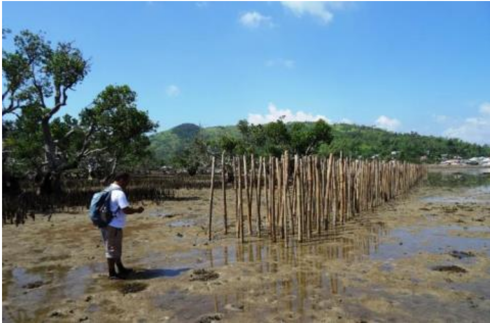
Figure 3: Bamboo breakwaters Ernesto Azuelo inspecting bamboo breakwater under construction in Igbon, Concepcion Municipality
