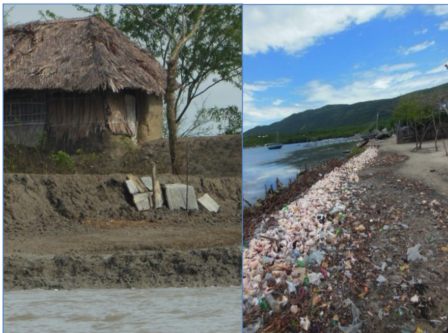
In each case residents have strategies in place to manage coastal risk. The picture on the left was taken in the Sundarbans. It shows a mud embankment with some concrete blocks for basic protection. The image on the right is of a shell and wood embankment that residents of La Gonâve have constructed to protect from erosion
