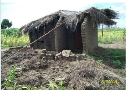
Zione's house, destroyed by heavy rains
