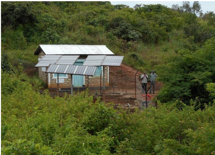
Figure 13. Solar pumping scheme installed in Ngara District by Concern.
