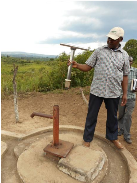
Figure 3. Broken hand pump at PE2.
