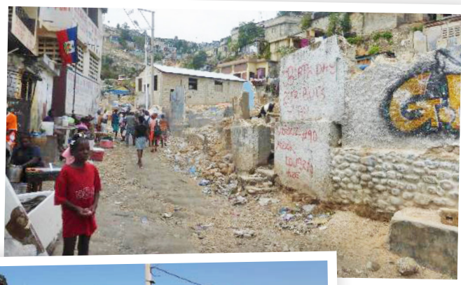
Before and After Picture of the Construction of the Ravine Vasquez in Grand Ravine. Photos Katia Antoine and Frederic Mogin
